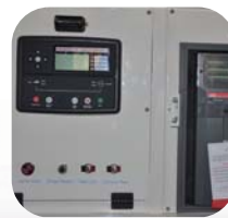
Control Panel & MCB
